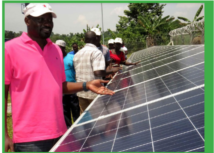
Solar panels powering Masulita piped water project
