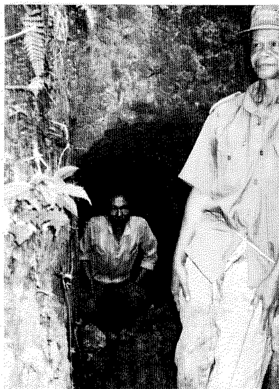
The Tunnel: a community initiative to dig through the hill and save on pipe costs.
