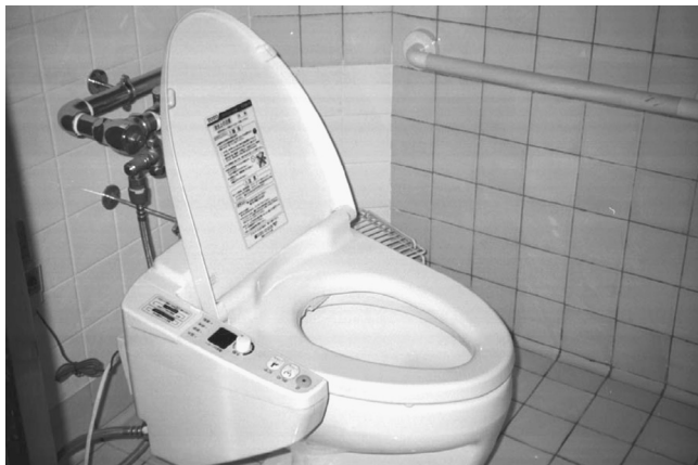
FIGURE 7. Electronic Sit-Down Public Toilets, Japan
