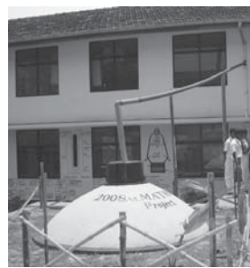
Partial under ground Ferro cement tank
