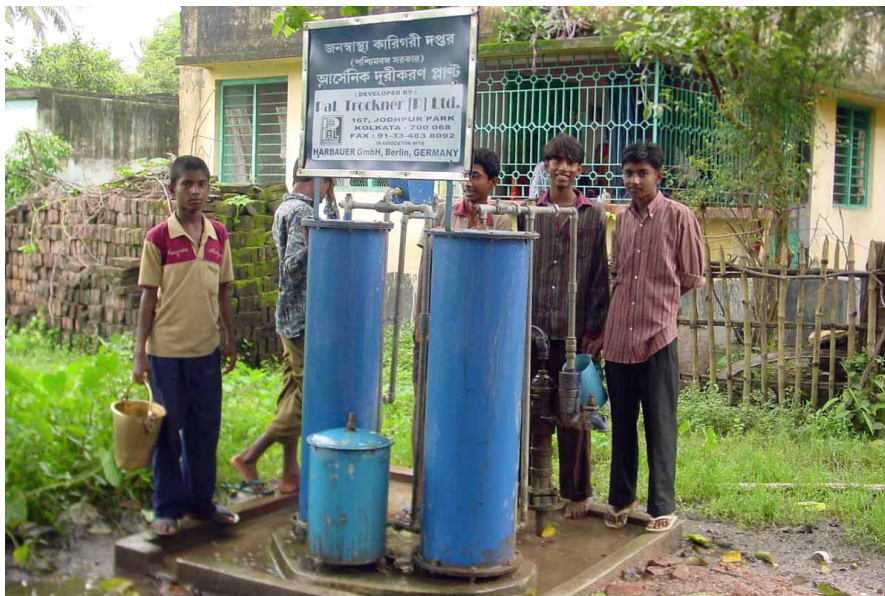
Figure 14: AdsorbAs ® arsenic removal plant in West Bengal, India. The plant is designed for a supply of up to 500 L/h flow rate.
