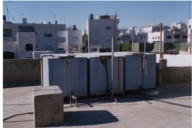
Above: Household rooftop storage for filling by connection or tanker
