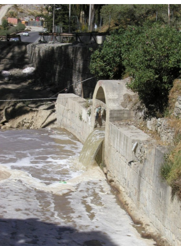
Wastewater discharge into rivers
