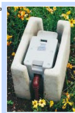
YARD METER ABOVE GROUND
