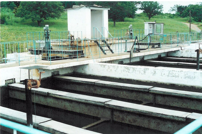
Treatment works, Zambia (NWASCO photo)
