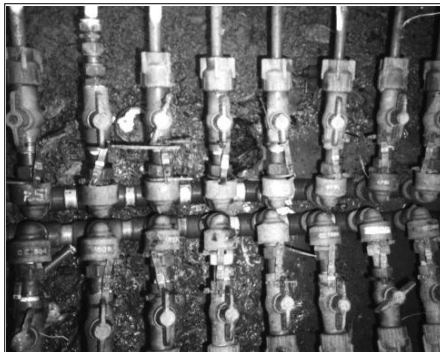
'Durban Tank': Manifold for daily household tank filling IMO Working Group, WSSCC, Kayaga Photos ↕
