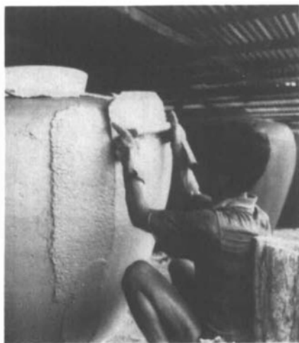
Two 20mm coats of cement plaster with reinforcement between them make up the walls of the jar
