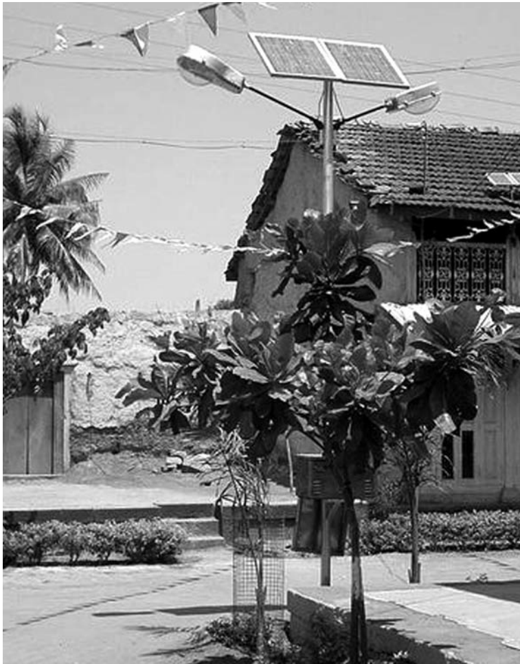
Figure 10.5 Solar street lamp
