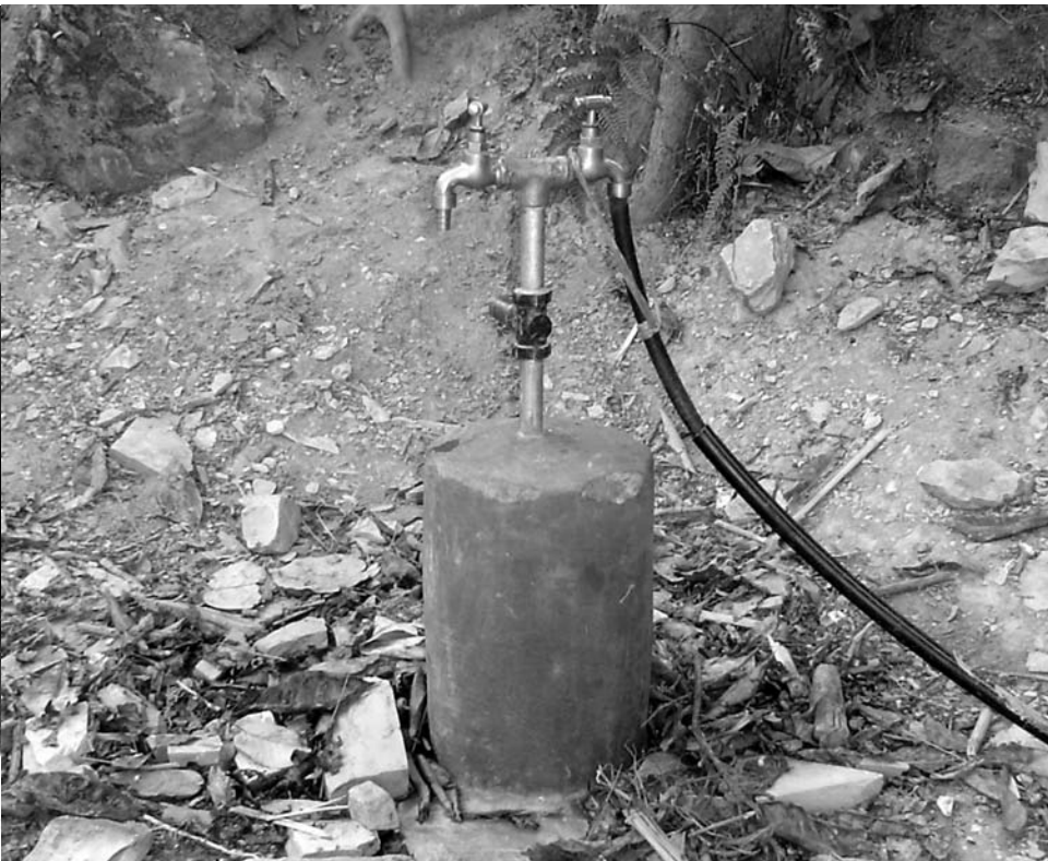
Figure 4.5b Irrigation offtake with hose attached to fill a drip header tank
