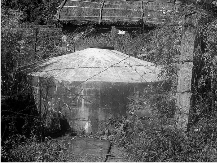
Figure 5.2 25,000 liter Mul Pani drinking water tank
