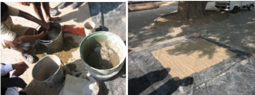
The cement paint is prepared and the hessian sheet laid on plastic sheet,
