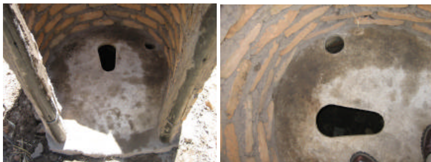
The arrangement of the slab and brickwork. Also the arrangement of the squat hole and the vent hole.
