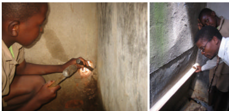
The PVC pipe is used as a urine collector and attached to the existing wall of the urinal. The pipe was 2.5m long made from 75mm PVC pipe. A section of 1.7m was cut out to form a channel in which the urine will flow. A hole is made in the external wall of the urinal and the pipe is placed along the existing urinal wall leading out through the wall to fit over the tank outside.
