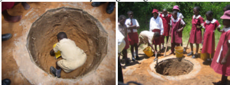
Pit being dug down to one metre depth and soil rammed around the ring beam
