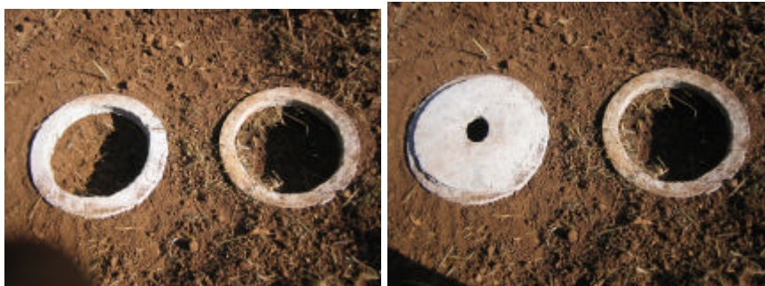
Two ring beams used in the Fossa alterna . Cast ring beams in place and when hard dig inside both down to 1.2 to 1.5m. Add a sack of leaves to the pit which is used. Fit the slab on one ring beam and cover the second for safety. The second can be filled with leaves and soil to make compost.
