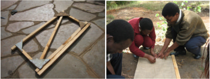
The door frame is made with wooden “brandering” and triangular plywood corners. A single diagonal strut supports the frame. Some form of covering is added to the frame. In this case sacking material called hessian.
