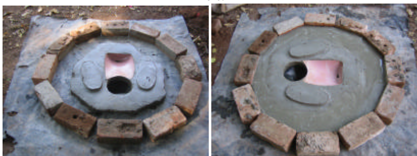
A circle of bricks is laid down around the slab to the required size. This is then filled with concrete with some reinforcing wire inserted. It is left to cure. This urine diverting slab offers a clean non absorbent surface for urine collection, which can be made at low cost.
