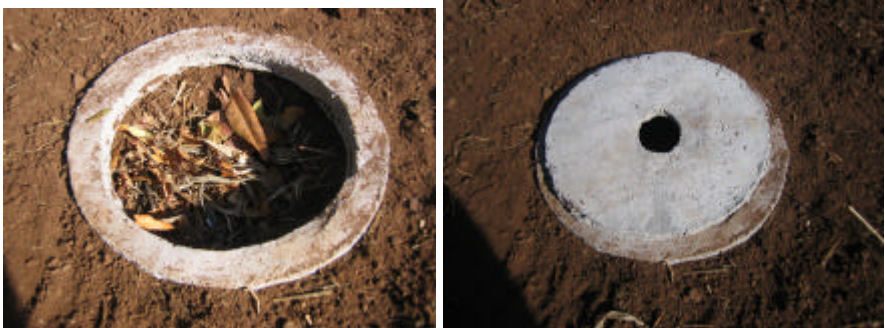
The ring beam has been cast on ground allowed to cure and a hole dug down inside. The slab has been fitted.
