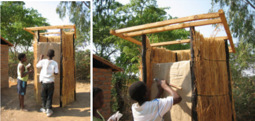
The hessian door panel is nailed to the door frame. This could be treated with cement paint later to make it more durable.
