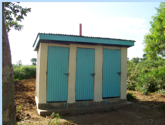
Figure 2. Latrines constructed with KESSP funds at DierAora Primary did not use the recommended KESSP design.
