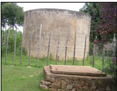
Picture 5. MG water supply reservoir
