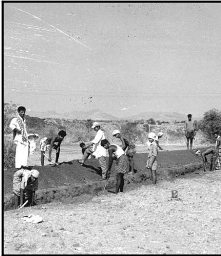
Male villagers work on a trench in the watershed village of Mucluikuatapalli
