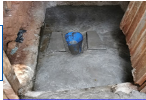
Fig-27: Common problems during Sato installation
