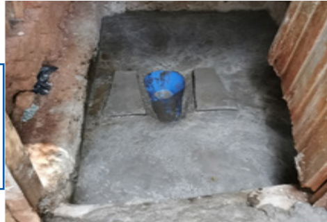
Fig-27: Common problems during Sato installation
