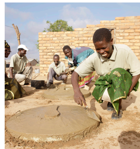
Elifa Mwaungulu, building a latrine slab, Chikompulazi village, Mzuzu, Malawi. Credit: WaterAid/Layton Thompson.
