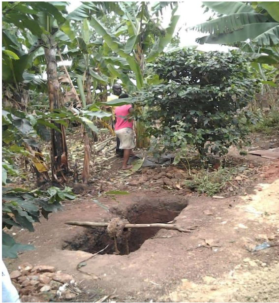
Excavation of a new latrine at the home of the LC1 chairman of Nyaruhanga village in Kasenda S/C
