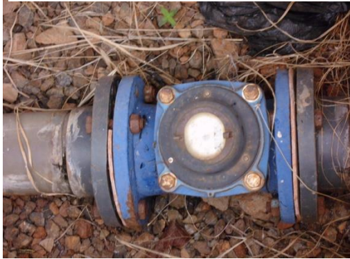
FIGURE 9: BROKEN BULK WATER METER
