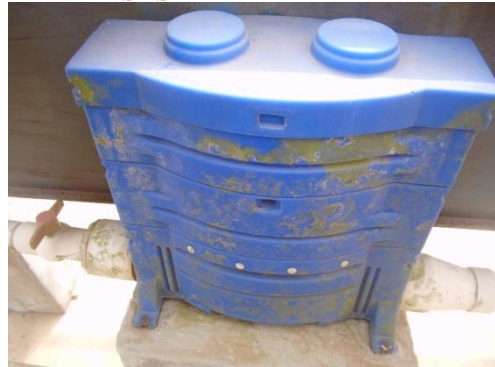
FIGURE 8: DISUSED CHLORINATION SYSTEM
