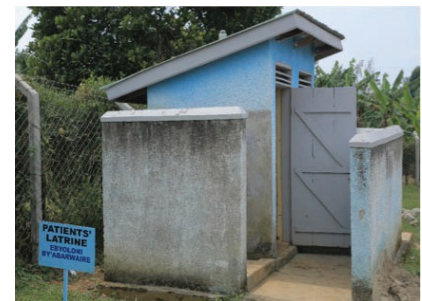
BEFORE: This unlined pit latrine has been the only available sanitation facility for all patients at Kaswa Health Center III in Kabarole.
