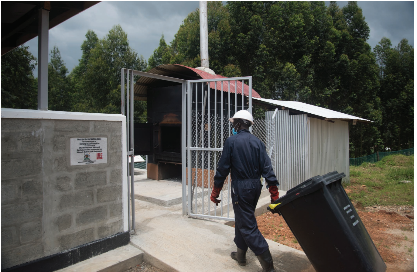
Healthcare facilities must have access to a licenced medical waste management facility such as this incinerator at Ruteete HCIII in Kabarole.
