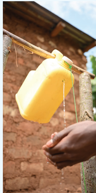
A tippy tap for handwashing locally installed near the latrine.
